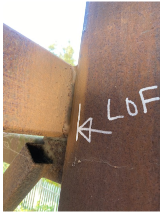
Rack 85, evidence showing lack of side wall fusion.
