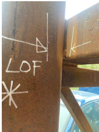
Rack 88 evidence showing lack of side wall fusion.
