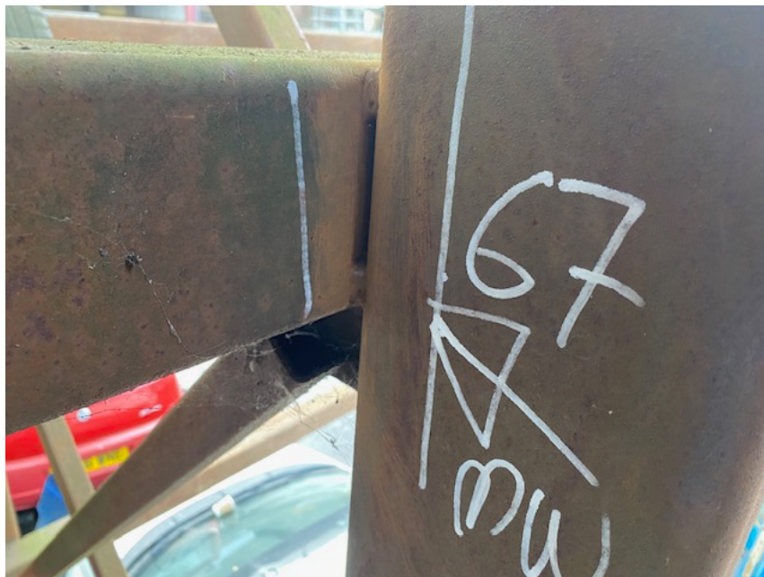
R67, Missing weld
