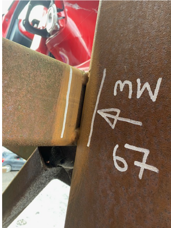
R67, Missing weld
